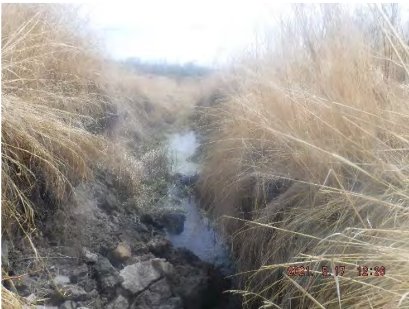
Photo 7: Erosion/slumping within ditch
