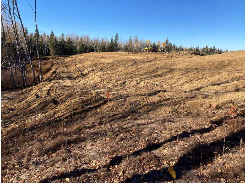
Photo 5: Photo taken looking southwest of the interim remediation of the erosion on the back of the south slopes.
