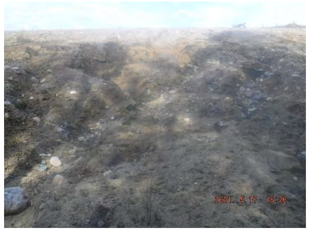
Photo 8: Erosion along the southwest boundary.
